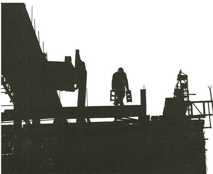
Worker walks atop the Fine Arts annex as it looked in February. —Photo by M. Brunner
