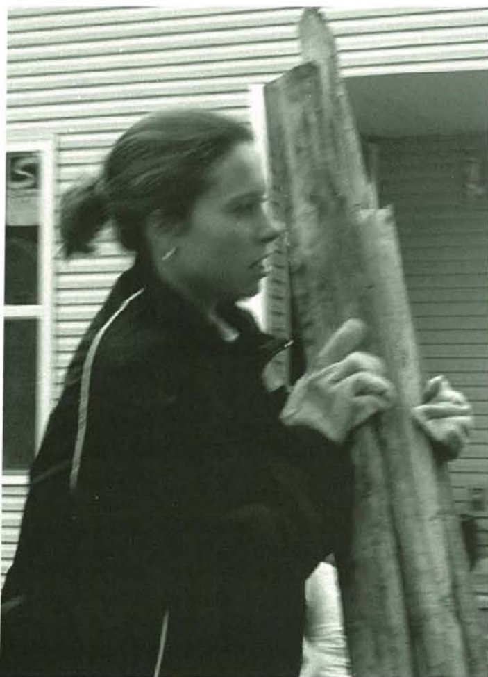
Anna Ristic cleans up debris at Habitat for Humanity. Habitat for Humanity helped build homes for lower income families.
