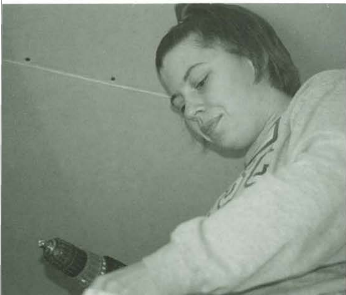
Top Left: Senior Jamie Florence drills for Habitat for Humanity. The group worked on hanging sheet rock for the house.
