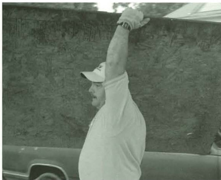
Don Willis carries siding materials to the work site. Final touches were put on one of the houses during "The Big Event."
