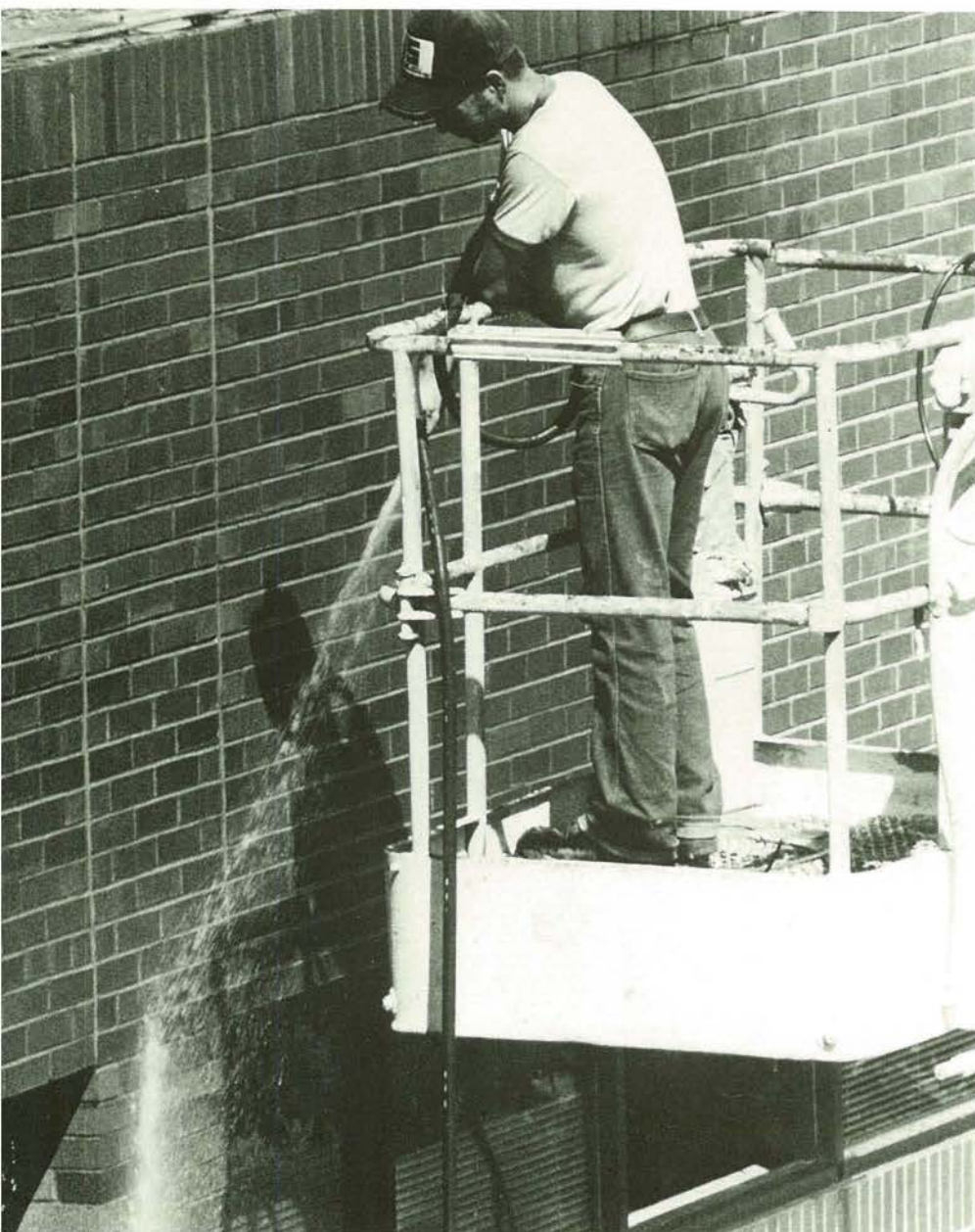
Member of the maintenance crew washes down the Building during the fall.—Photo by D. Logan
