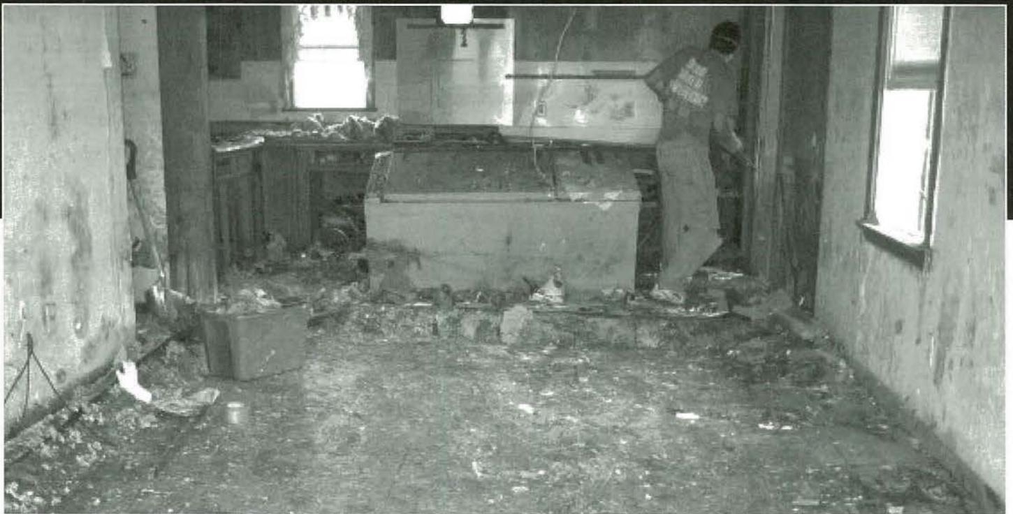
One student cleans up the kitchen of a house that was ruined by the disastrous Hurricane Katrina. Millions of houses were destroyed by the hurricane. Photo submitted by Trevor Parker
